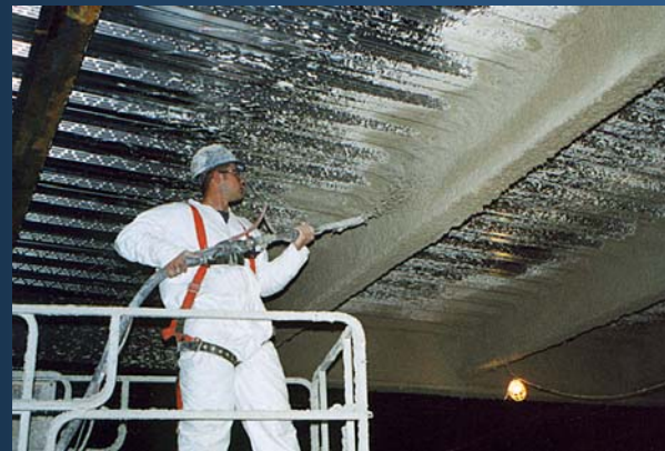
Spray-On Fire Resistant Material (SFRM)
